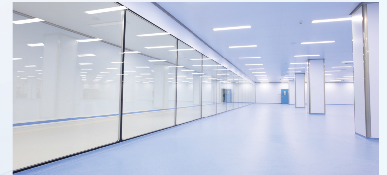
Clean room and HVAC
